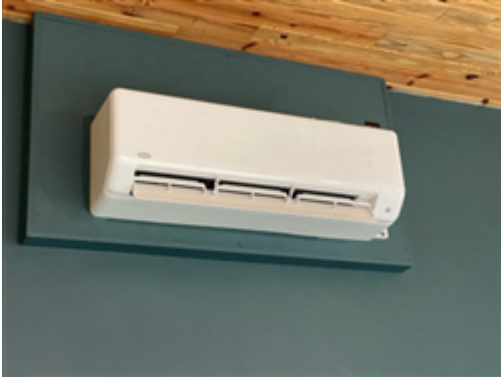
Photo - Heating and Cooling (interior) Unit #5
