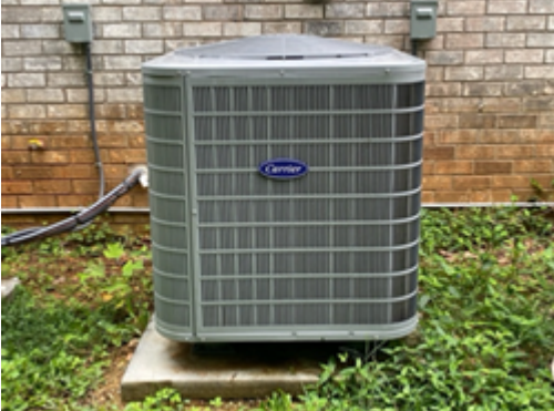
Photo - Heating and Cooling (exterior) Unit #2
