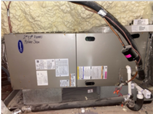
Photo - Heating and Cooling (interior) Unit #4
