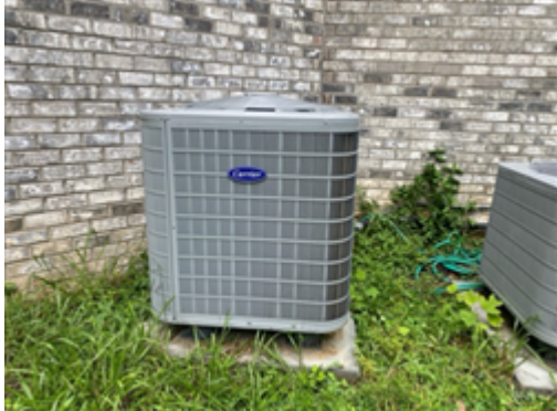
Photo - Heating and Cooling (exterior) Unit #1
