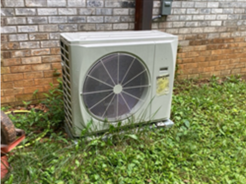
Photo - Heating and Cooling (exterior) Unit #5
