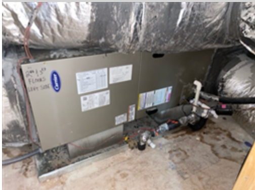
Photo - Heating and Cooling (interior) Unit #3
