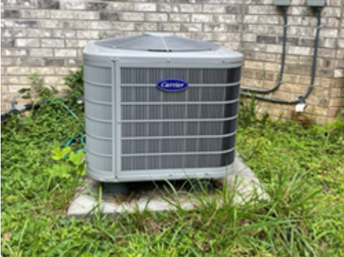
Photo - Heating and Cooling (exterior) Unit #3
