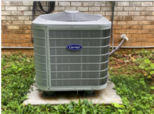
Photo - Heating and Cooling (exterior) Unit #4
