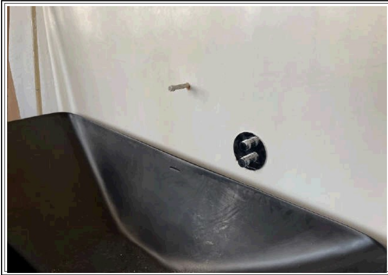
Primary Bathroom Tub missing faucet
