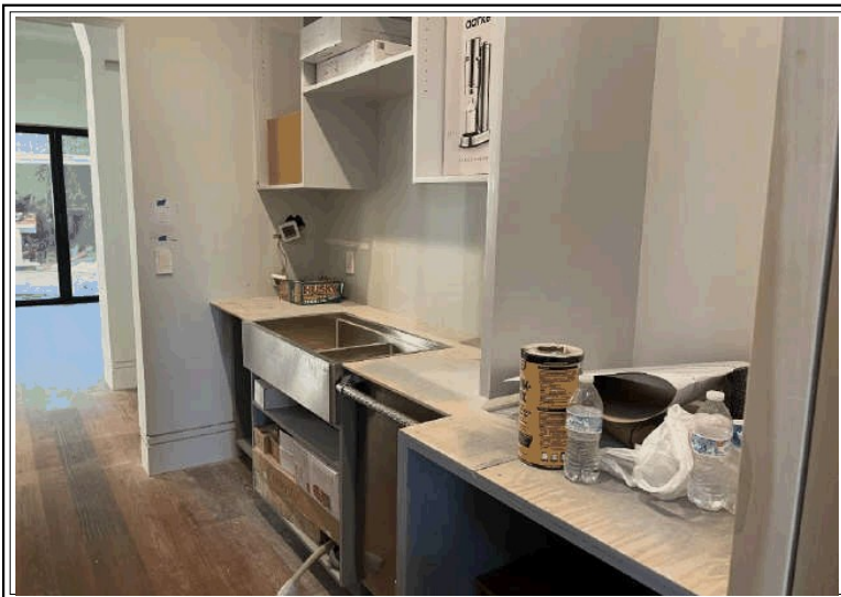
Wet Bar Missing cabinet doors and countertops
