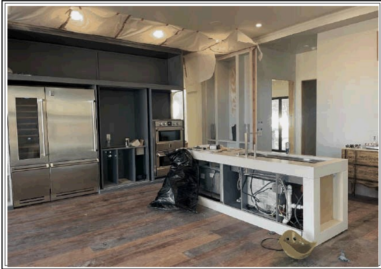
Kitchen Missing Doorfronts and Island Panels
