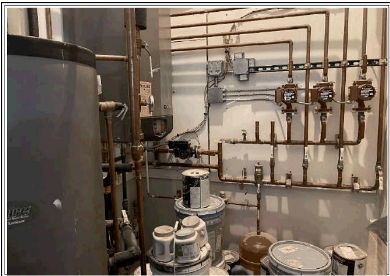
Radiant Flooring System & Hot Water Heaters
