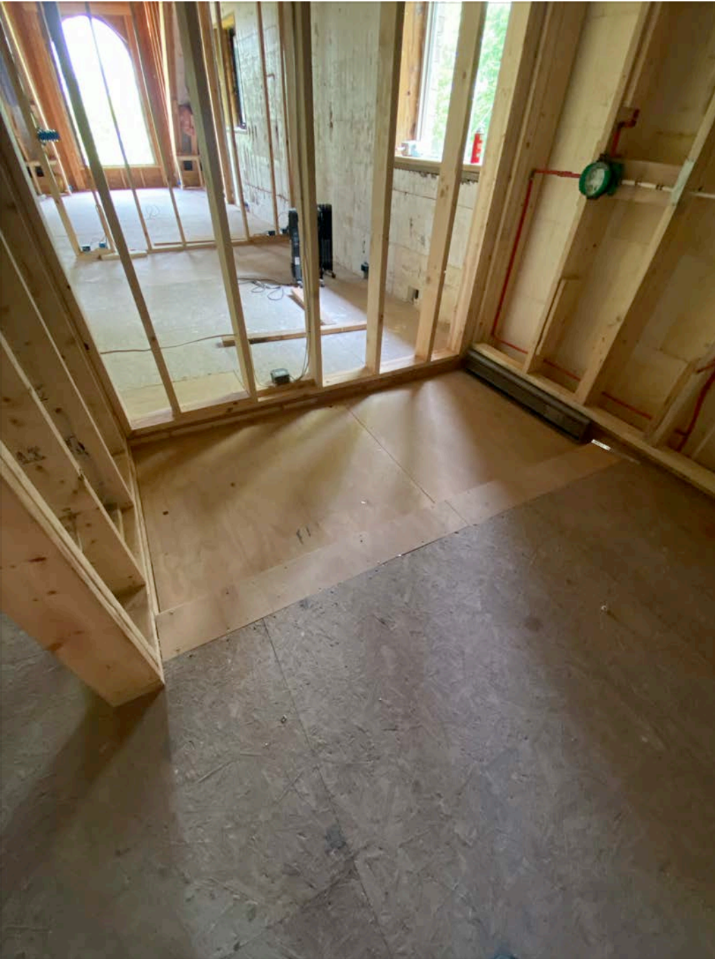
Plywood for walk in shower. Support underneath already logged in master closet. Bathroom wall shared with room 9 2x4 and frame kit for pocket door
