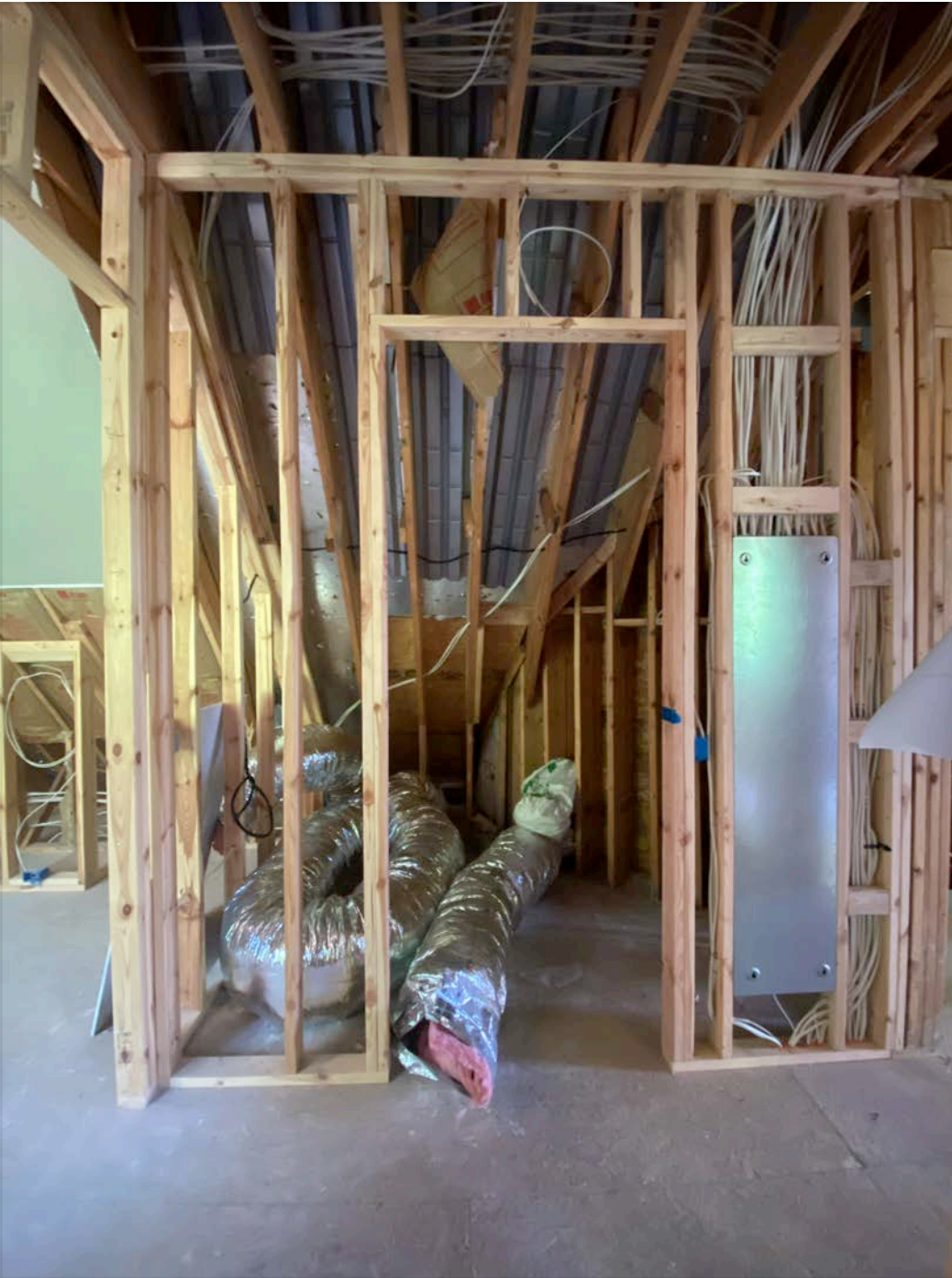
Bathroom back wall with plumbing (redone twice and molded boards partially removed and replaced after homeowner complaint) 10 2x6, 9 2x4
