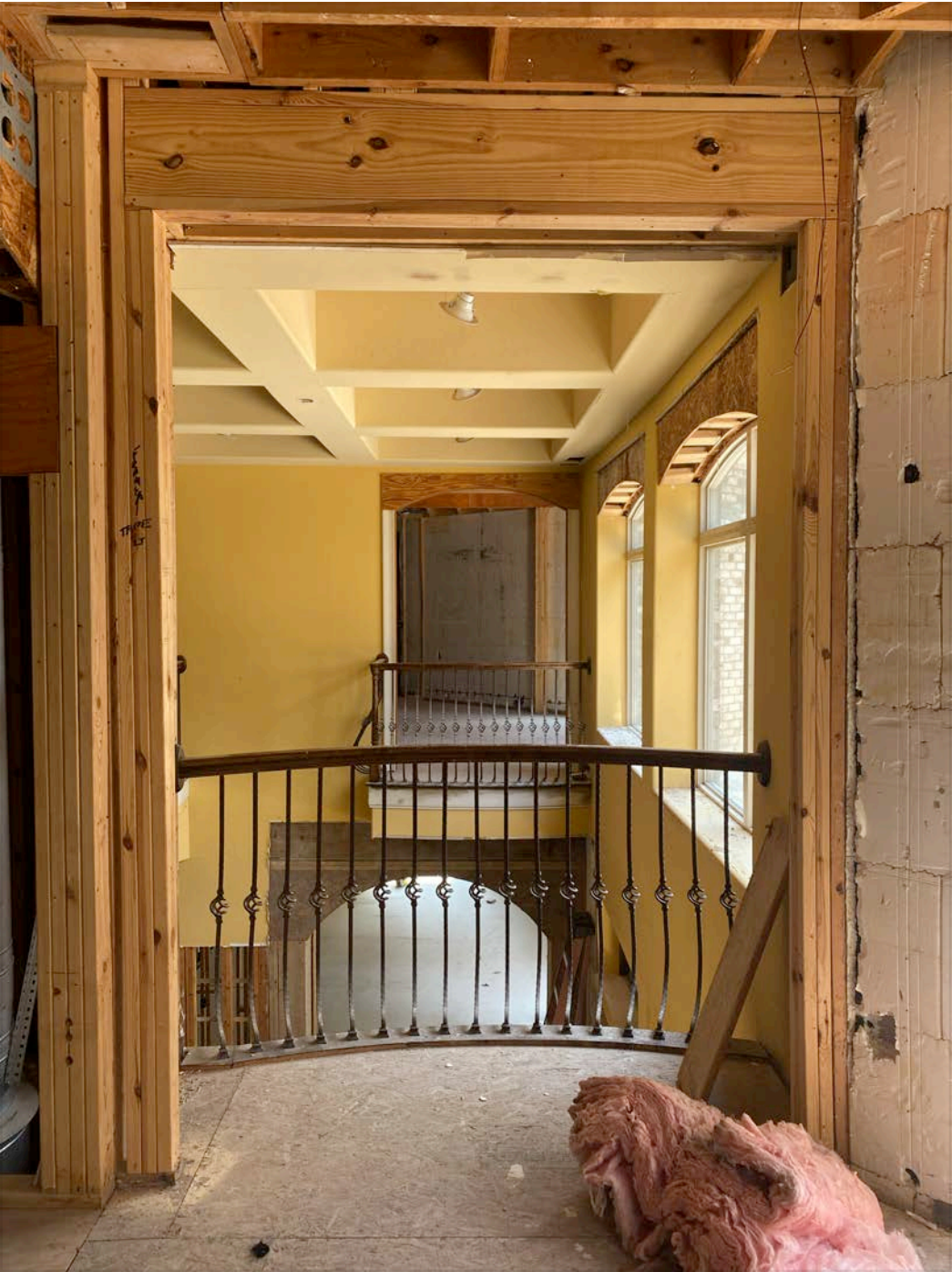
Partial of wall and arched entrance to office from studio: 12 2x4 and 2 2x10
