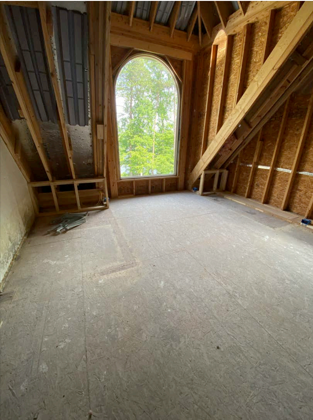
Diagonal reinforcement and window boxing: 6 2x4 2 2x6 for window boxing pictured below, diagonal wall reinforcement at 7 2x4 long, and 2 long 2x8 Lumbar for around window
