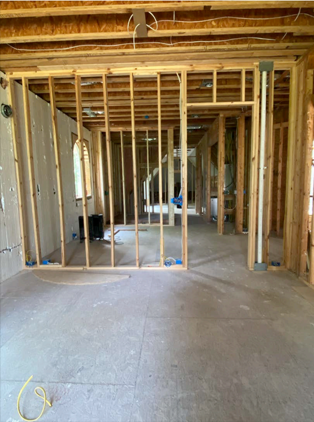
Wall between bathroom and lounge area (initially improperly framed with 2x4s reframed with 2x6 and still not showing area for niche).
