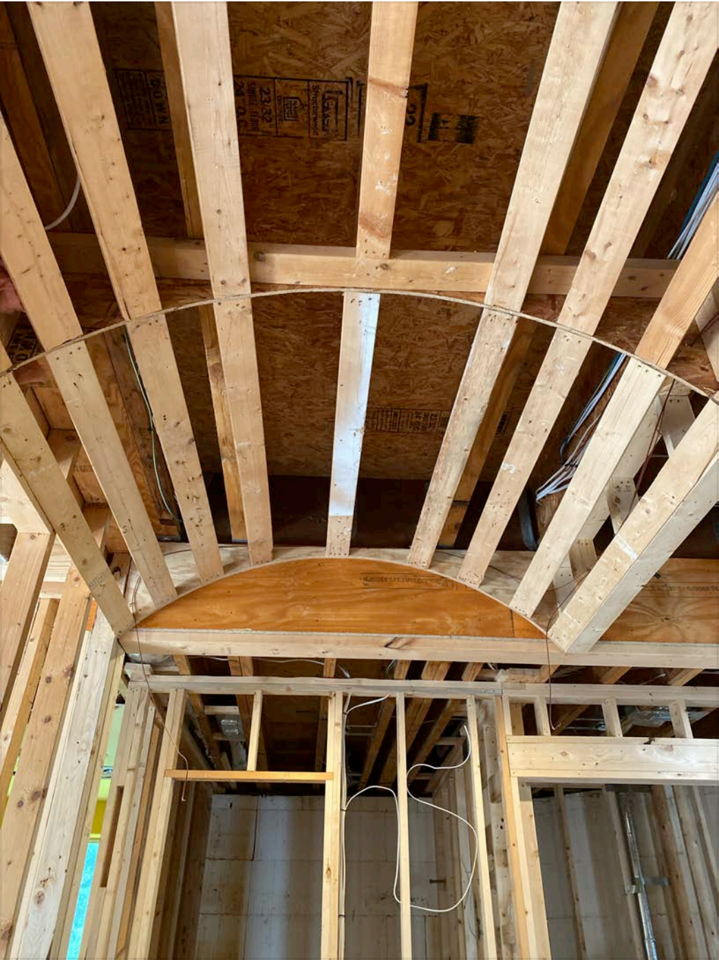
Arch of barrel opposite side by Angela's office: some arched sheathing and less than one 2x6
