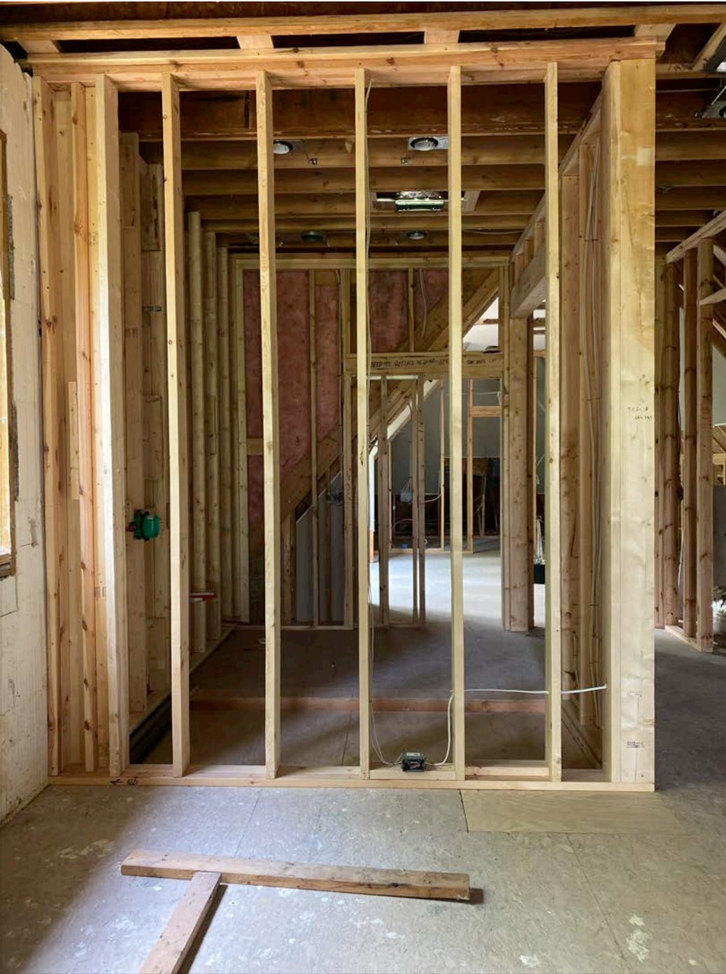
Hallway wall shared with bathroom that contains doorway area to bathroom: 15 2x6
