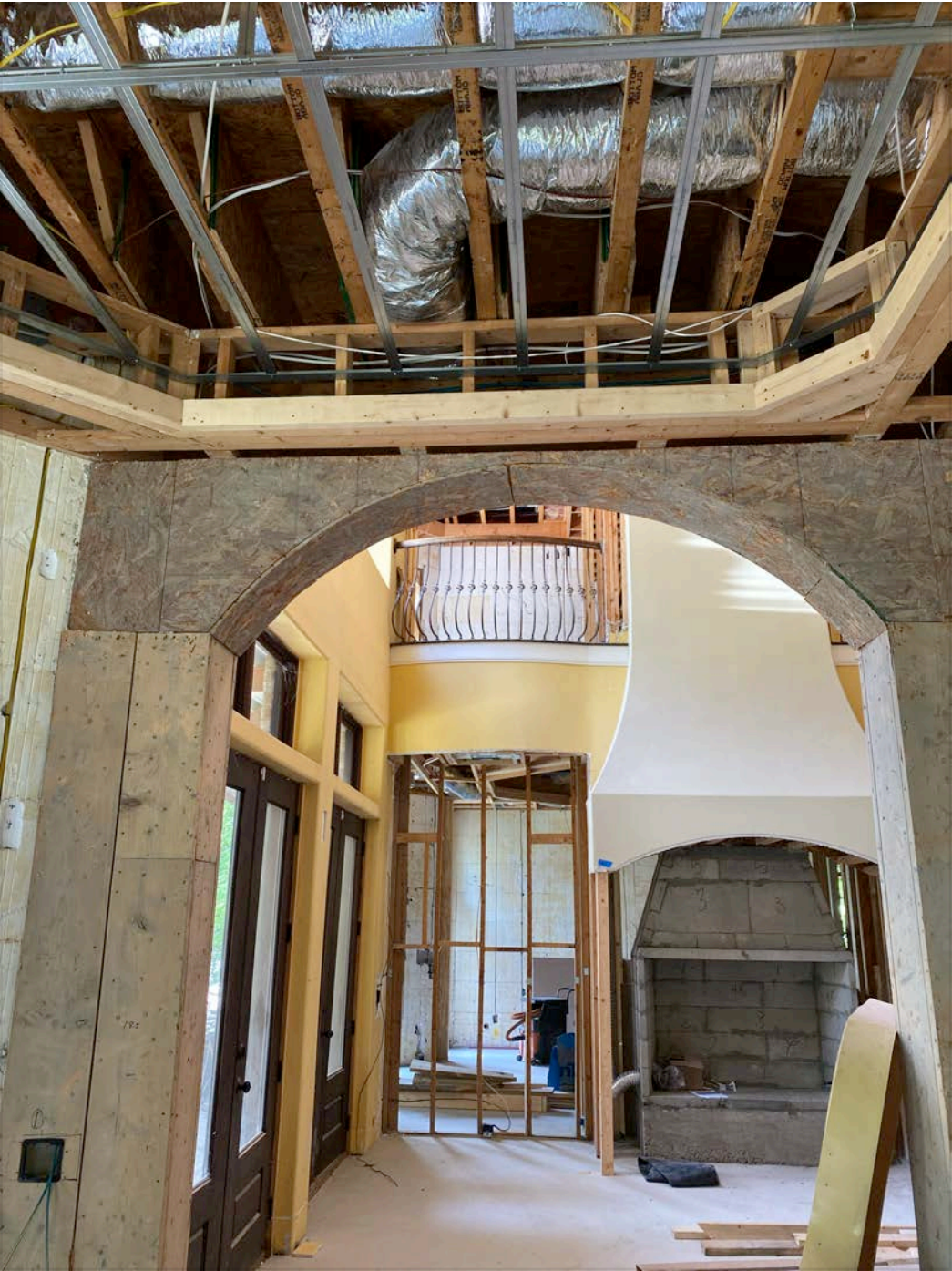
Ledge for tape lighting over arch to great room 7 2x4 Ceiling Edgework over pantry entrance 6 2x4
