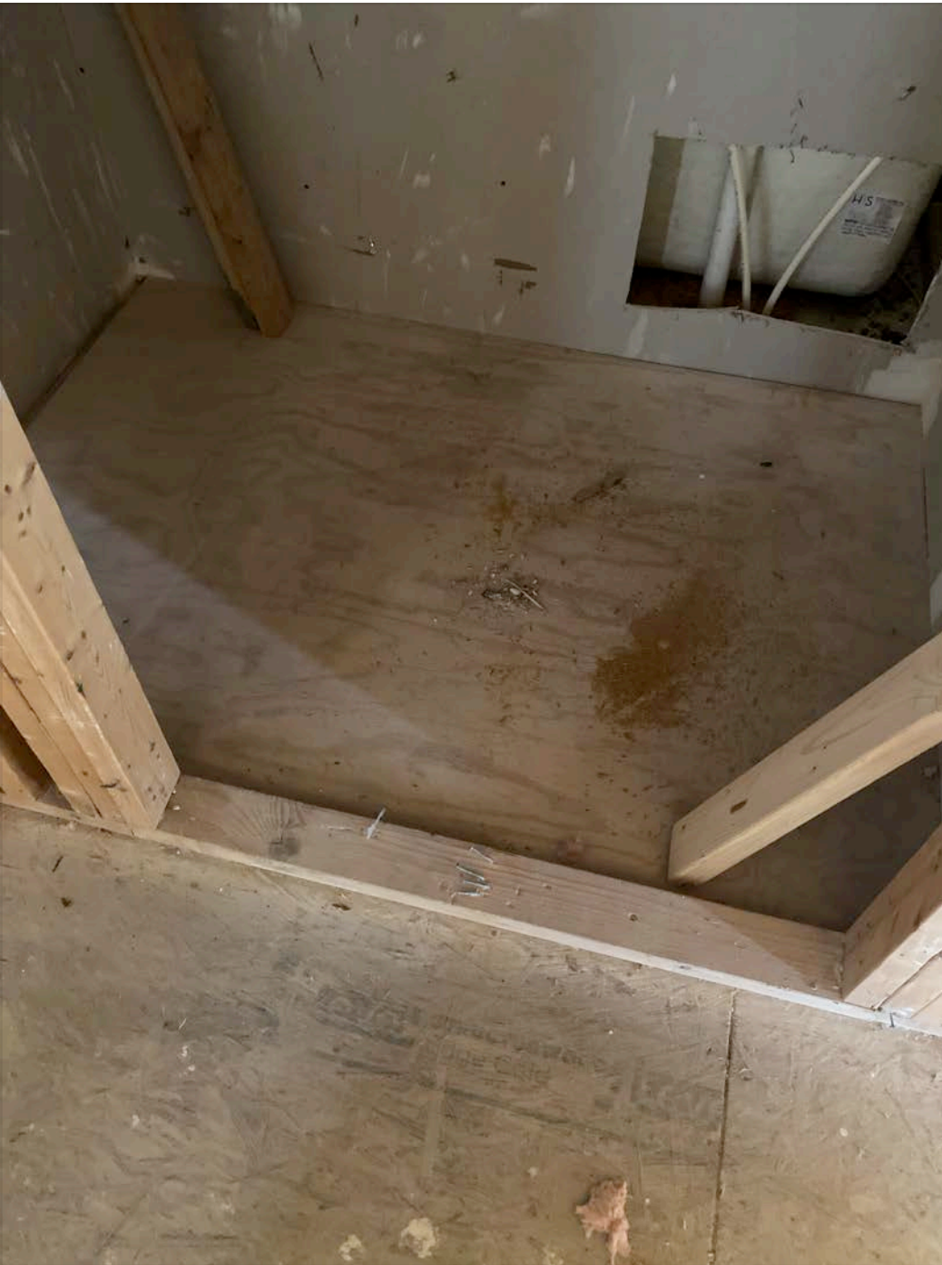
Second level bathroom shower floor: qty 2 Misc patches on second floor: no more than 6 qty
