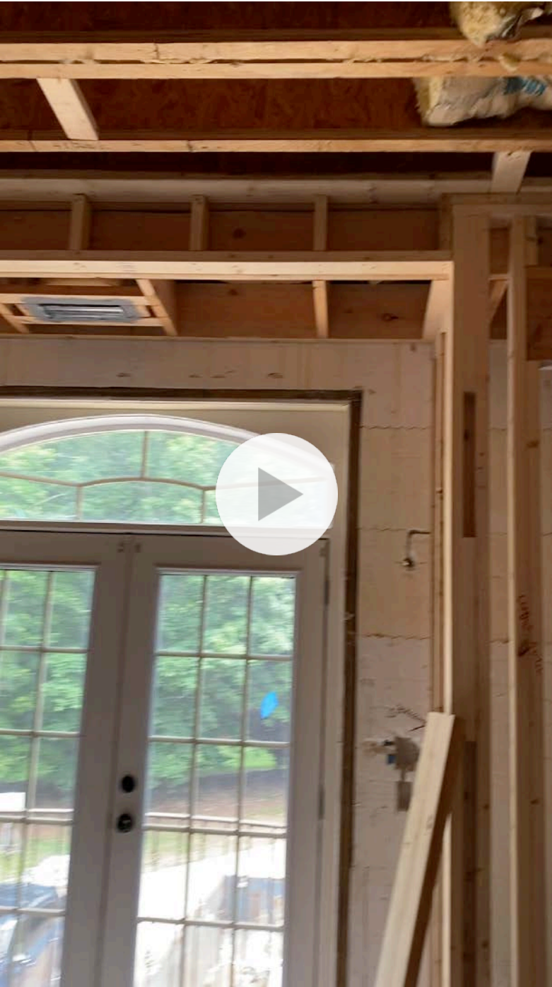
2nd floor elevator closet 3 2x4 and whatever was used for floor (sheet plywood)
