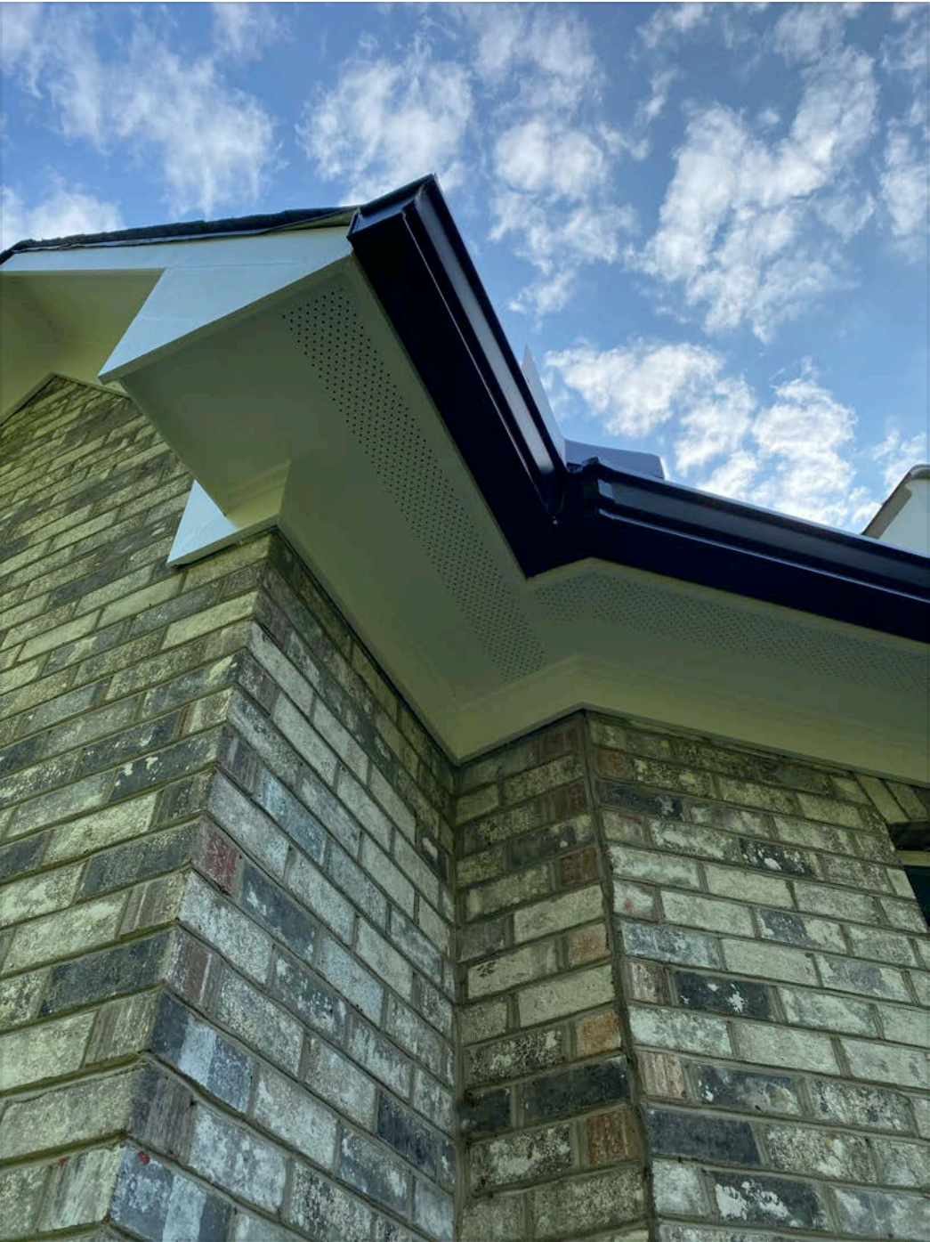
Examples of paint job poor quality for soffits and fascia:
