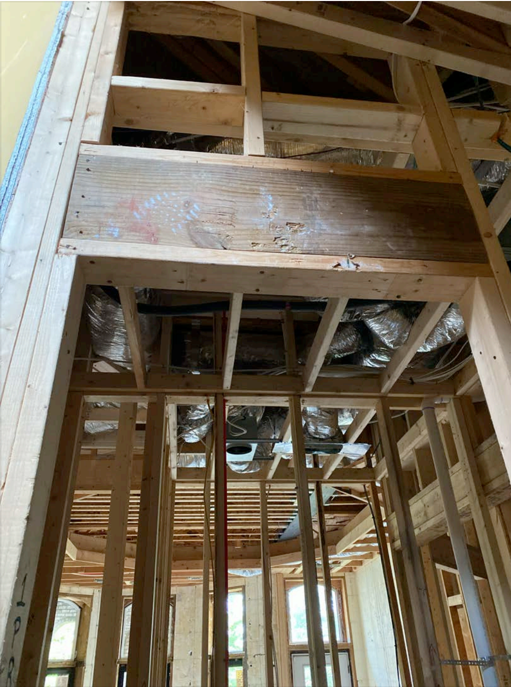
The engineered beam in the fireplace area is not sized appropriately to the space and the area is not framed in a way that sufficiently supports the load above (according to the neighborhood architect I brought in who looked at it):
