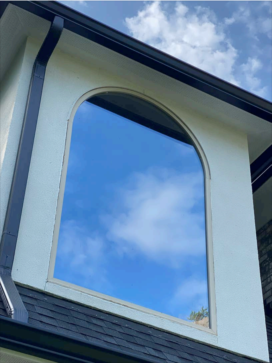
Difficult to see in this particular photo, however caulk separated
