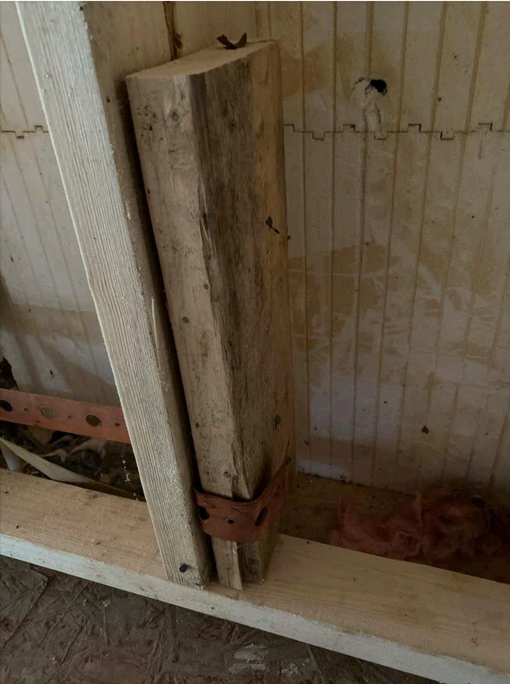
Moldy boards used in framing of guest bathroom
