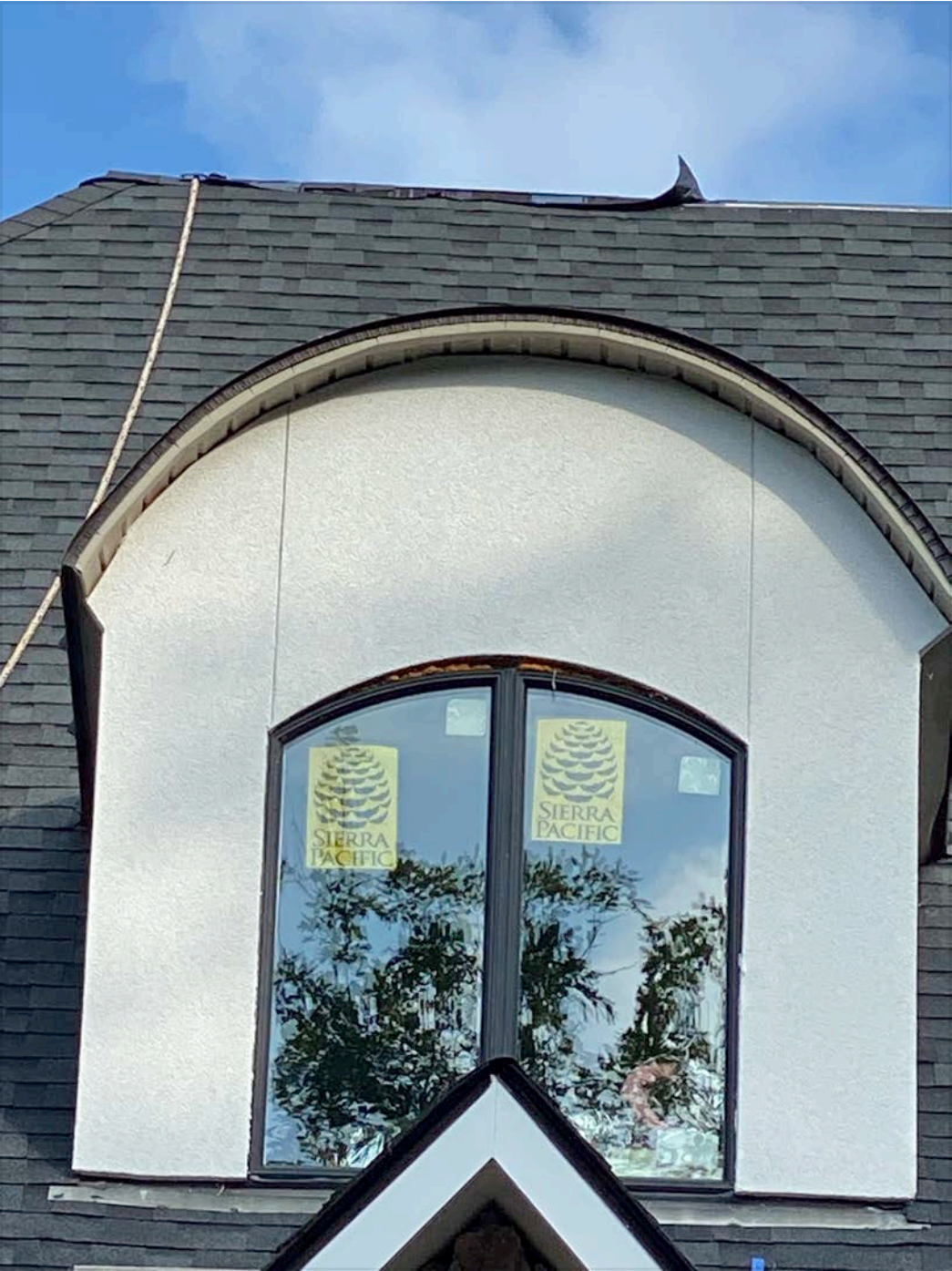
Old miscolored curved venting/soffit with gap underneath:
