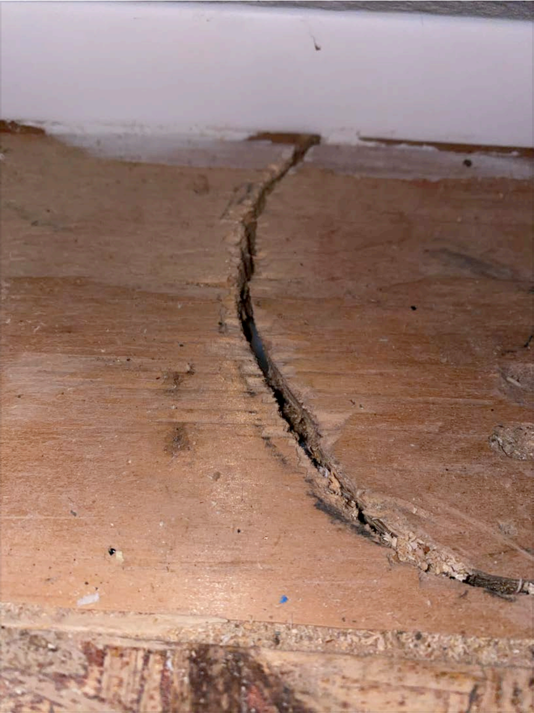
2nd floor bathroom toilet drain not secure
