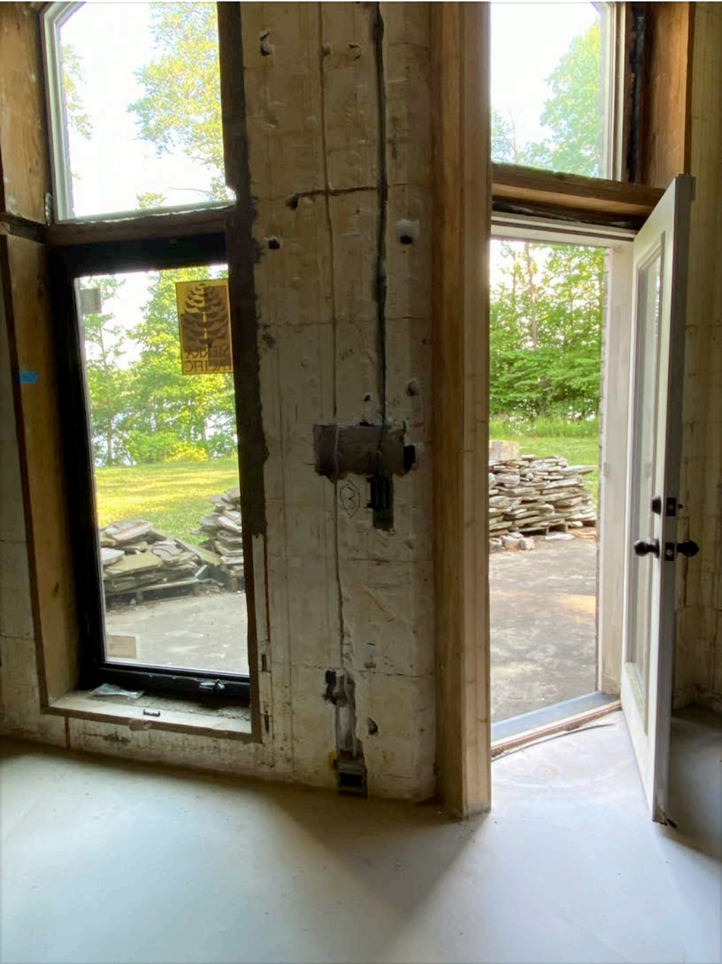
Art room sink plumbing installed too close to end of wall due to miscommunication by project manager to sub:
