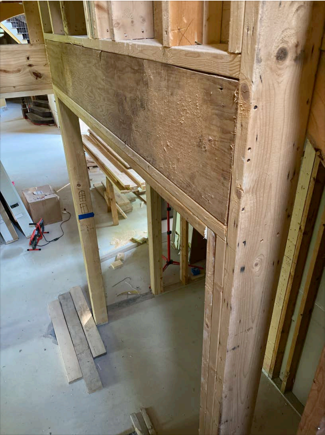
Moldy boards used in pantry entry framing
