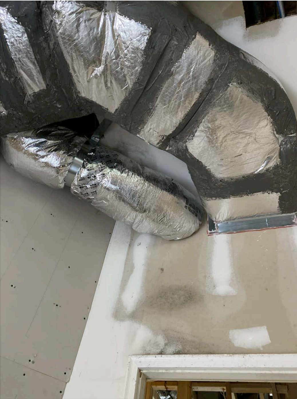
Multiple areas of home still evidence mold which must be fully remediated prior to drywall.
