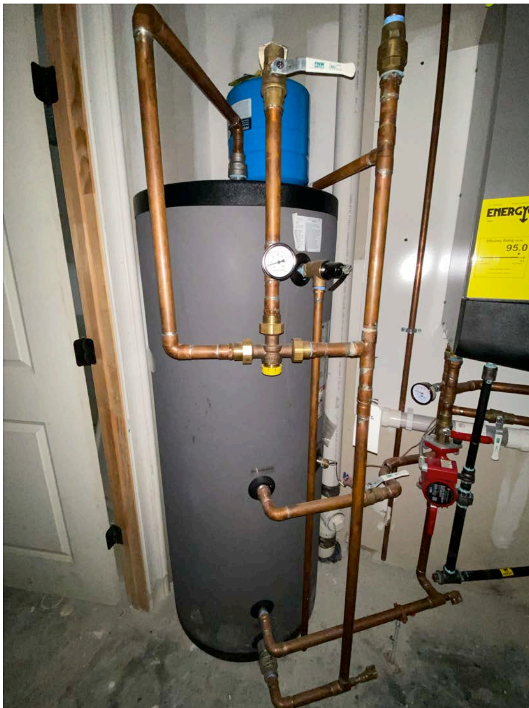
James B agreed to Angela that he would prep this wall prior to this install so the pipe work would look impressive. Instead, no prep was made to wall and misc cut pieces were put behind gorgeous copper work. Sad.
