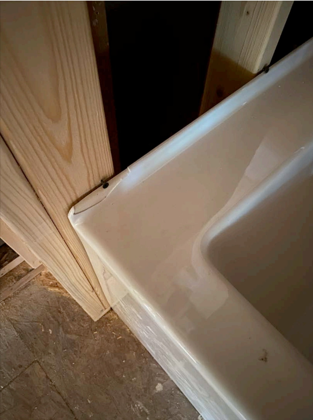
Third floor shower pan installed over circular cut portion of mismatched subfloor without consideration of adjacent marble flooring and what is necessary to exist underneath to support that:
